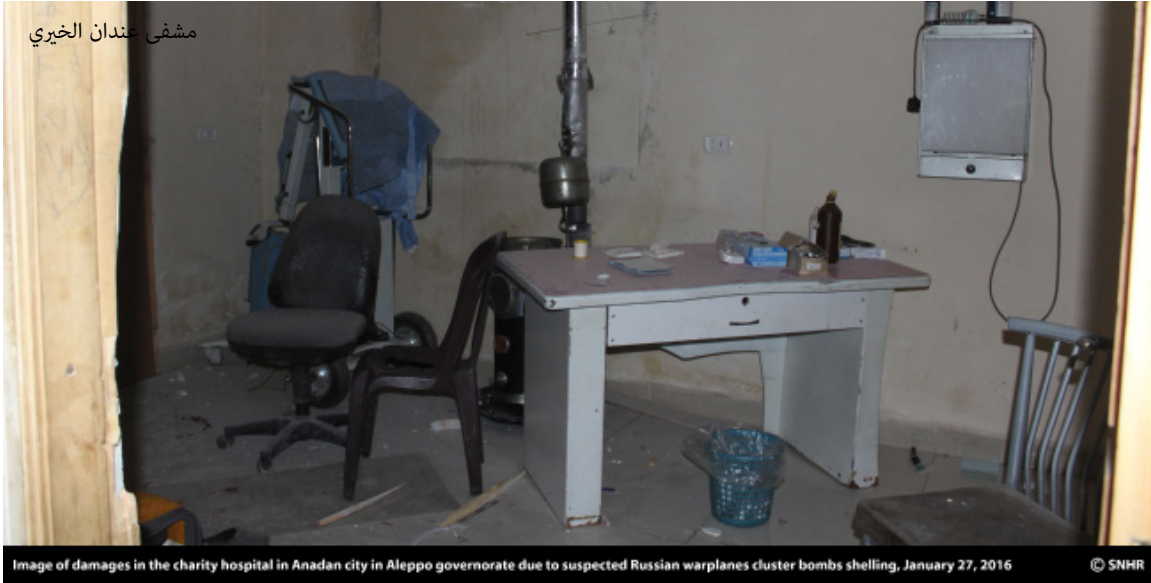
Image of damages in the charity hospital in Anadan city in Aleppo governorate due to suspected Russian warplanes cluster bombs shelling, January 27, 2016
