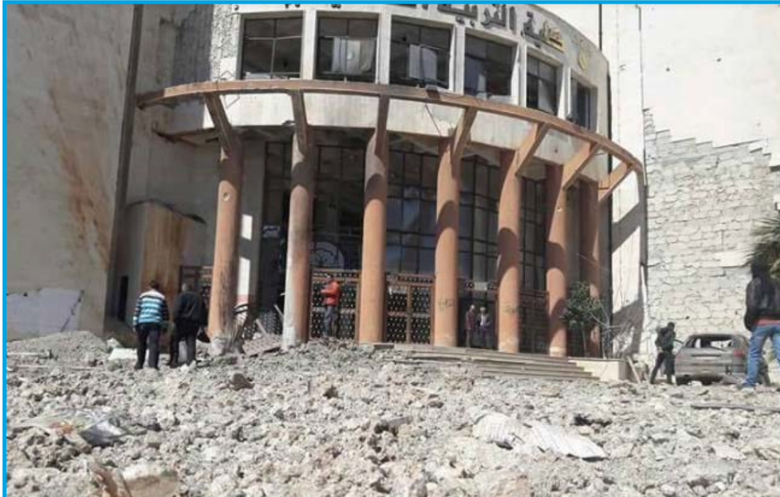
The destruction of the main gate of the education college after a bombing by fixed-wing warplanes we believe were Russian, Idlib city – March 25, 2017
