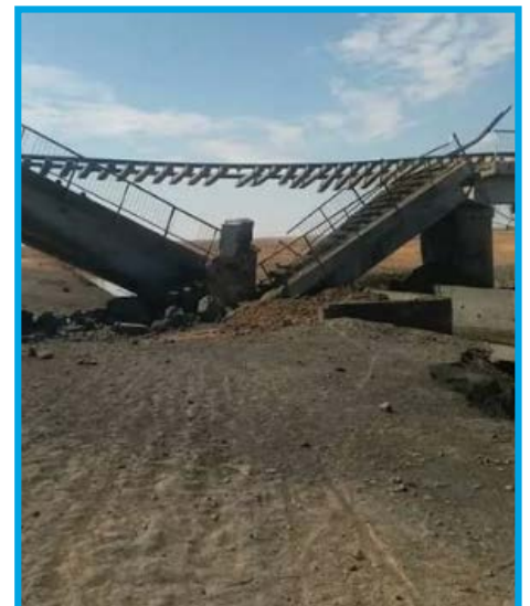
The destruction in the railroad bridge in the aftermath of a bombing by fixed-wing warplanes we believe were Russian in Rasm al Faleh village, Aleppo – March 23, 2017
