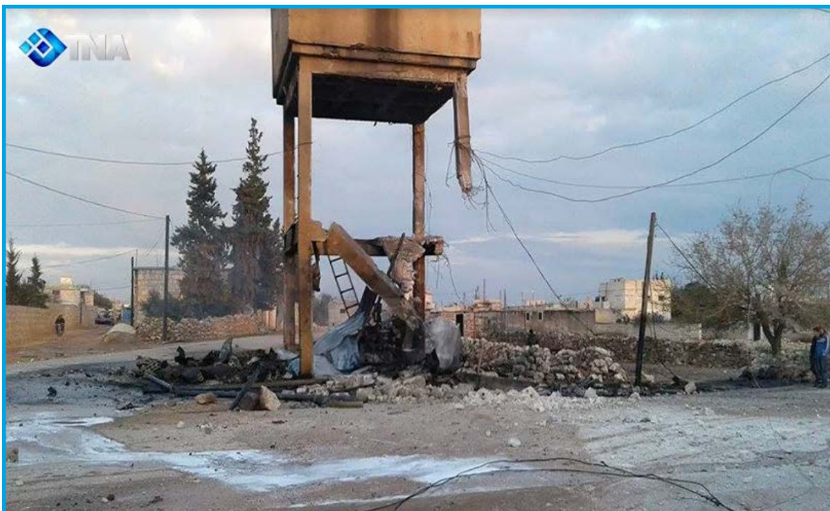
The destruction in the high water tank in the aftermath of a bombing by fixed-wing warplanes we believe were Russian, al Sheikh Ali village, Aleppo – March 16, 2017
