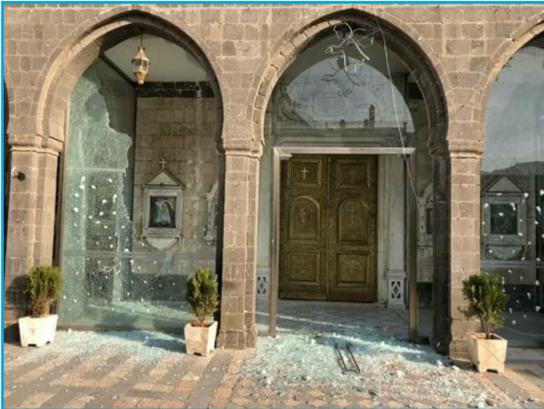
Damages after a rocket shell of unknown source landed on Sayda al Nayyah Cathedral, known as al Zaytoun Church, in Bab Sharqi neighborhood, Damascus – January 9, 2018
