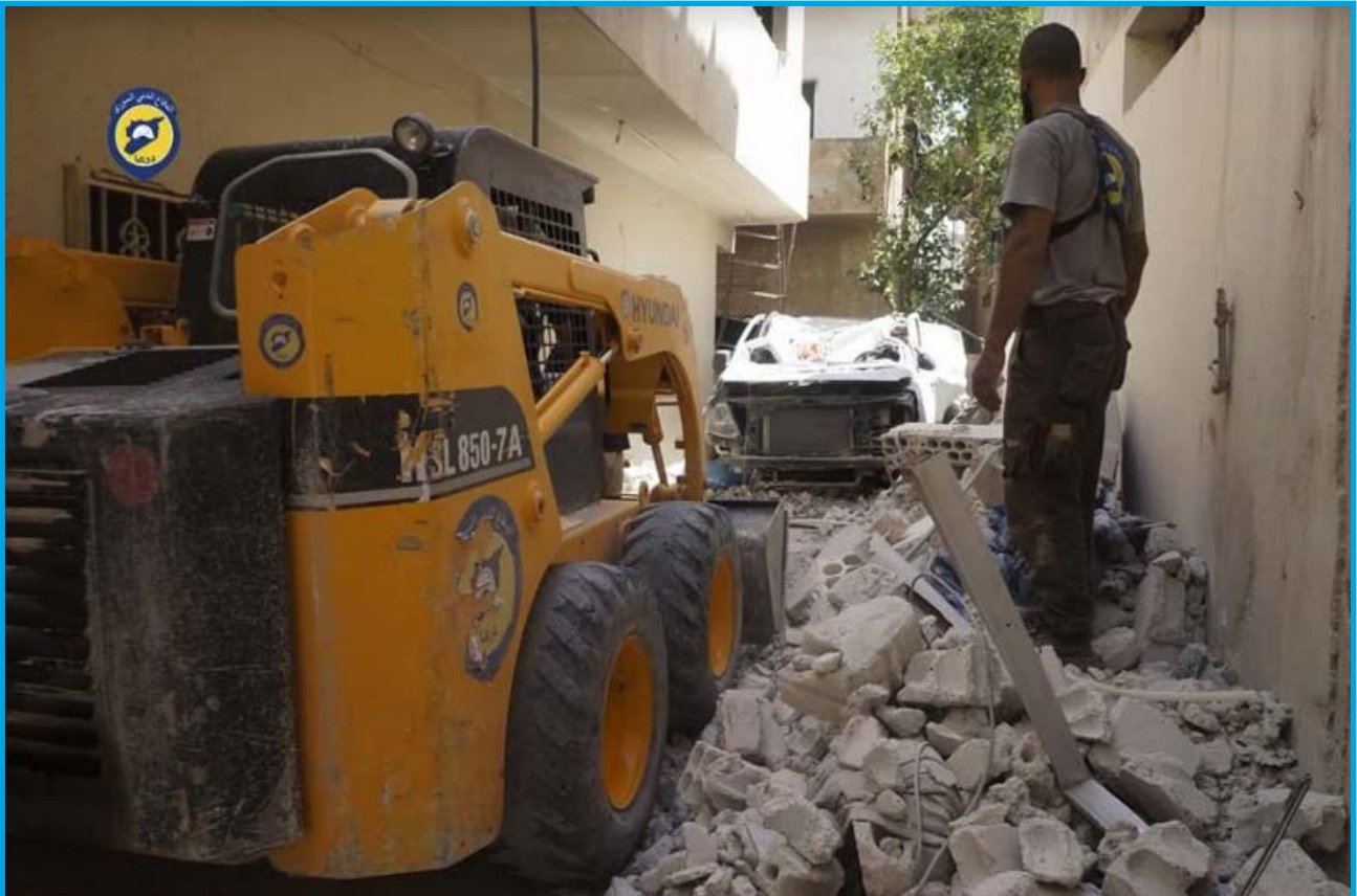
Damages resulting from a shelling by Syrian regime forces on center 1, which is affiliated to the civil defense, in Tareeq al Sad neighborhood, Daraa – June 12, 2017
