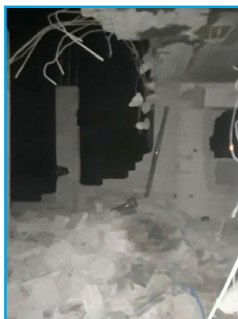
Destruction in the aftermath of a bombing by warplanes we believe were Russian that fired missiles at Kafr Zita Hospital in Kafr Zita, Hama – April 7, 2018
