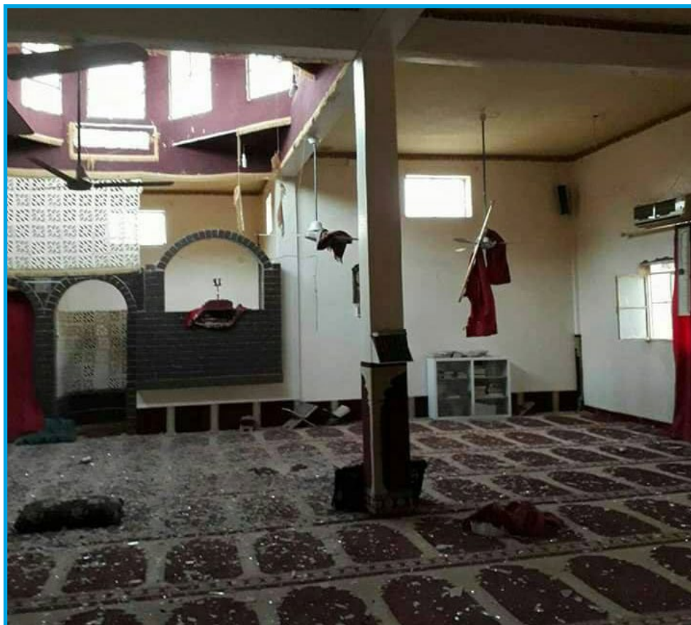
Damages in al Nab'iya Mosque in the aftermath of an air attack by Syrian regime warplanes, al Salihiya village, Deir Ez-Zour – November 3, 2017
