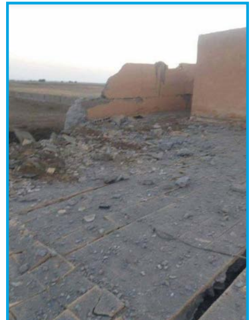
Damages in the aftermath of a Syrian regime bombing on Bedan School in Graniij city, Deir Ez-Zour – September 30, 2017
