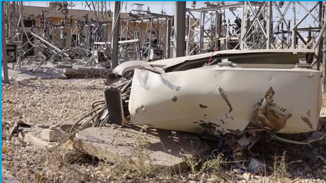
Damages at Khan Sheikhoun Substation in the aftermath of a Russian forces bombing in Kafr Ein village, Idlib – September 21, 2017
