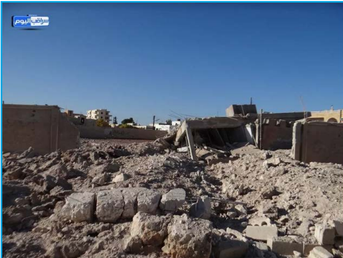
Damages at Hitteen School in the aftermath of an attack by fixed-wing warplanes we believe were Russian in Saraqeb city – November 17, 2016
