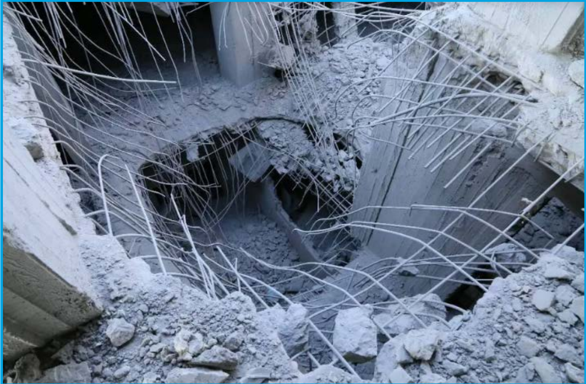
Destruction in the aftermath of a bombing by Russian forces on Sham Central Hospital in Kafr Nabbol city, Idlib suburbs – September 26, 2017
