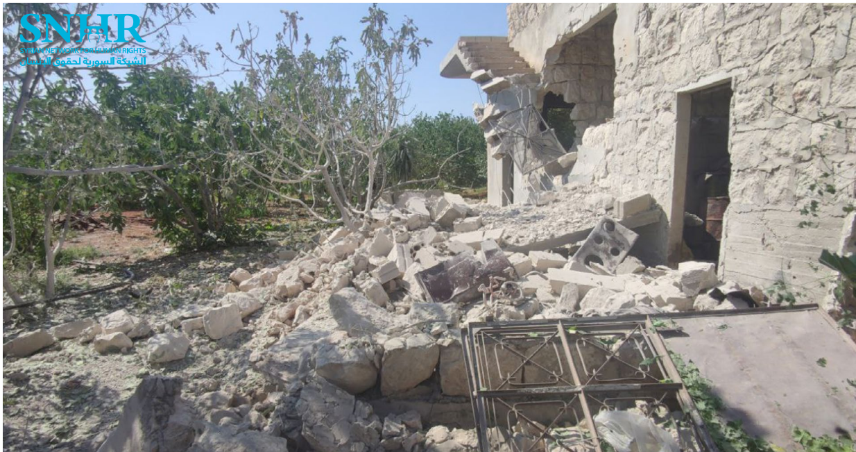
Damage to a house following shelling by Syrian regime forces in the southern outskirts of Shannan village, west of Idlib, on 6 September 2022
