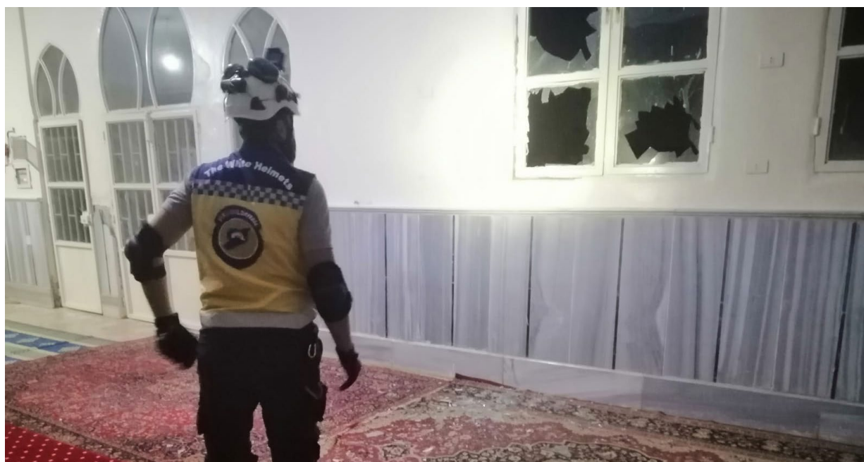
Damages caused by bombardment by unidentified perpetrators on Omar bin al Khattab Mosque in Uleshli village in Aleppo on September 15, 2022
