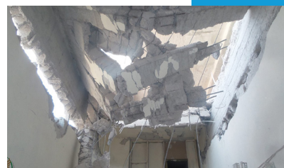
↑ 👁 Destruction caused by a Syrian regime barrel bomb attack on Nabd Houran Hospital in Dael city in Daraa - August 31, 2014
