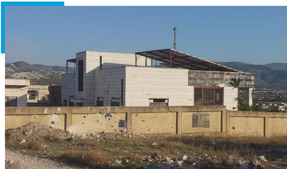
Ⓜ ↑ Damage following a Russian air raid near the dispensary in Bdama town in Idlib October 6, 2023
