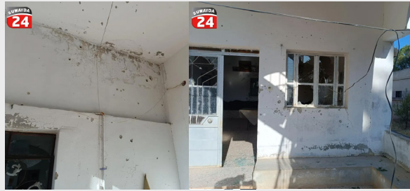
↑ Damage to a house in the town of Taara in the western countryside of Sweida as a result of mortar shells falling - June 5, 2025.
